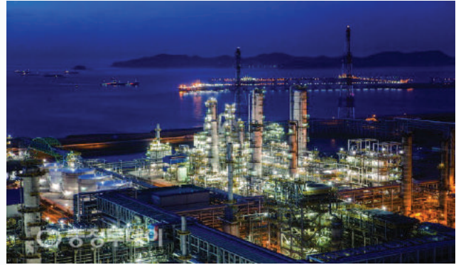
Lotte Chemical Industry 1300RT 3units, 975RT 1unit
